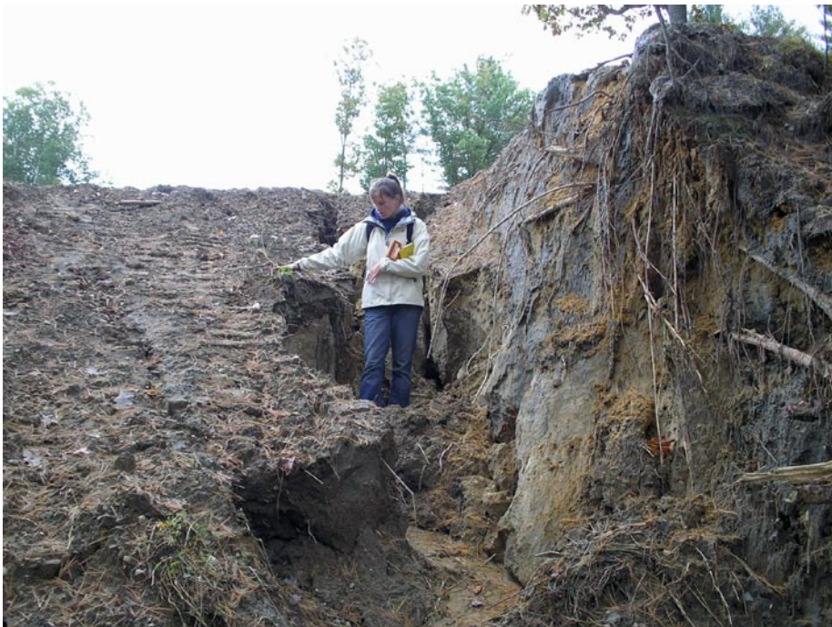
Effects of storm water erosion on steep slopes. Photograph courtesy of NHDES.
